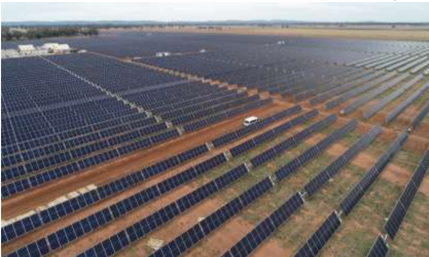
Jemalong 50MW Solar Project
