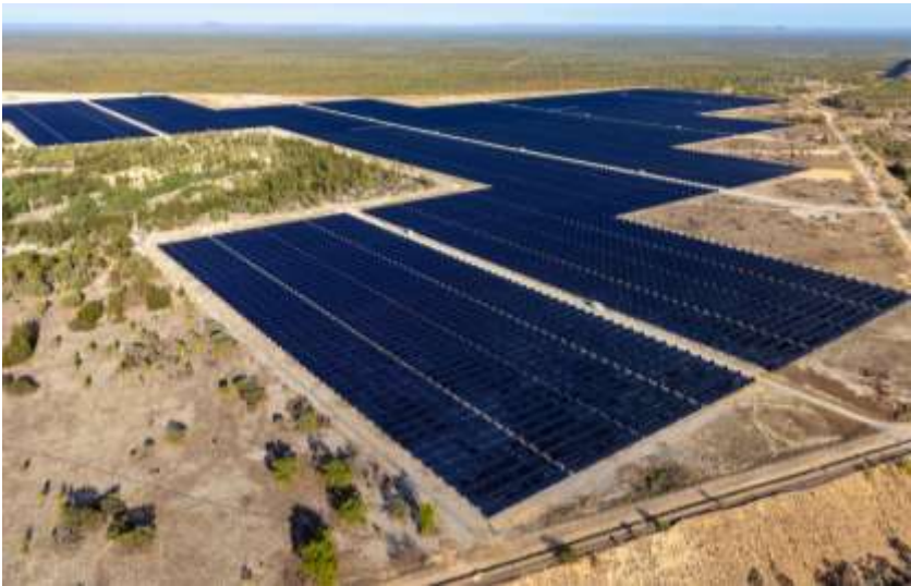
Kidston 50MW Solar Project
